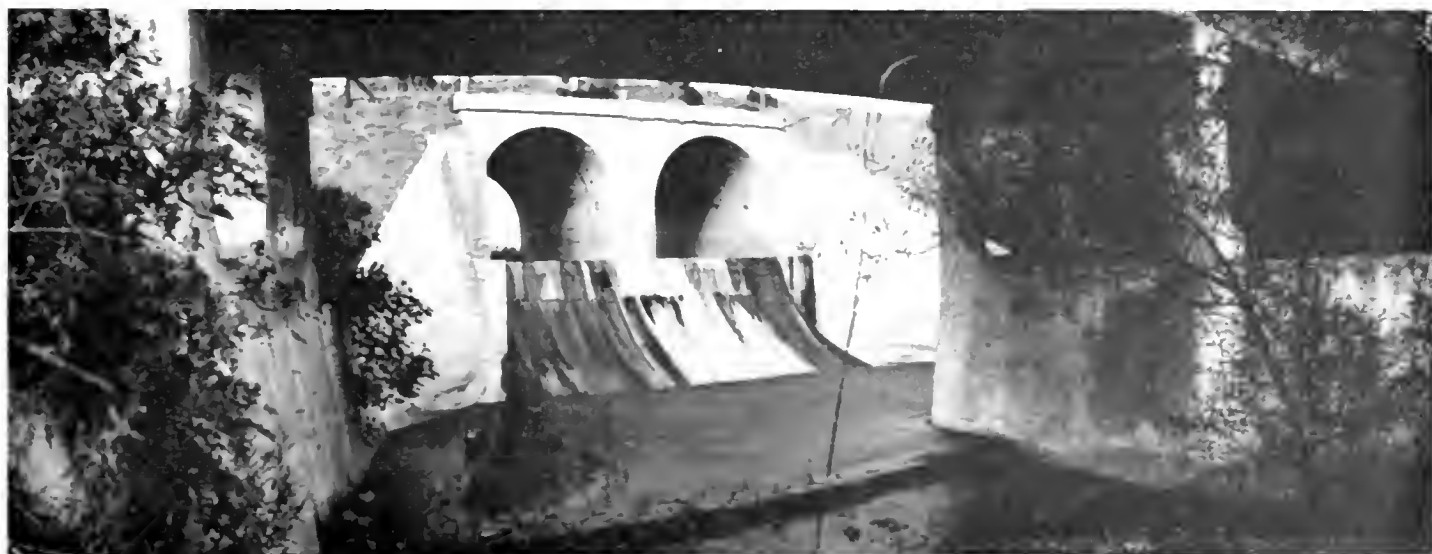
FIG. 56. Las Flores Creek. Looking under bridge at double arch culvert of A. T. & S. F. Railway
